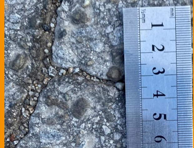
the control measurement shows 2 mm crack width that is clearly captured in the orthophoto
